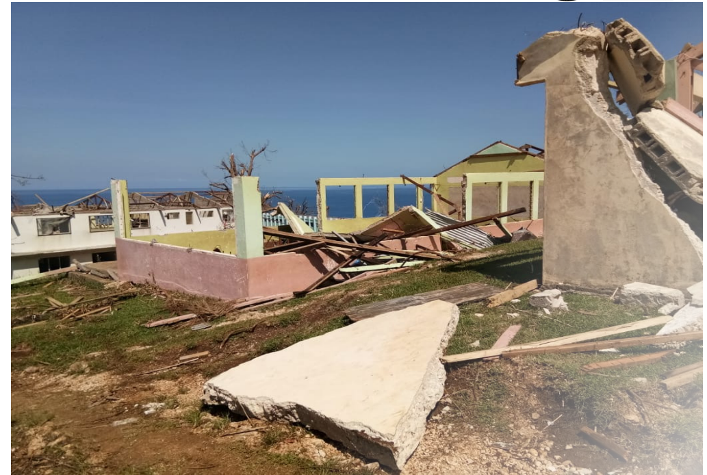
Source: IOM. Damaged building in Melsisi, Pentecost.
