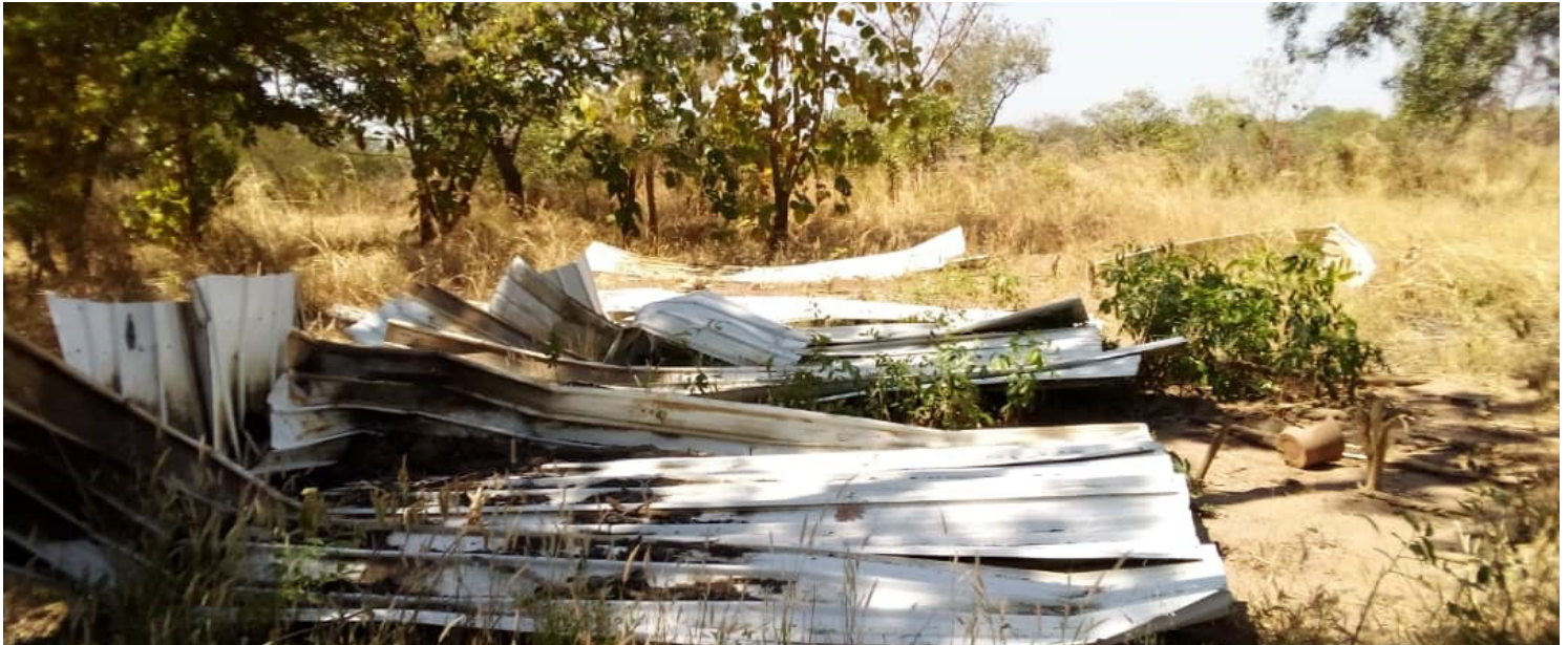
Kaabi collapsed primary school of Beselia payam of Wau county © IOM 2019
