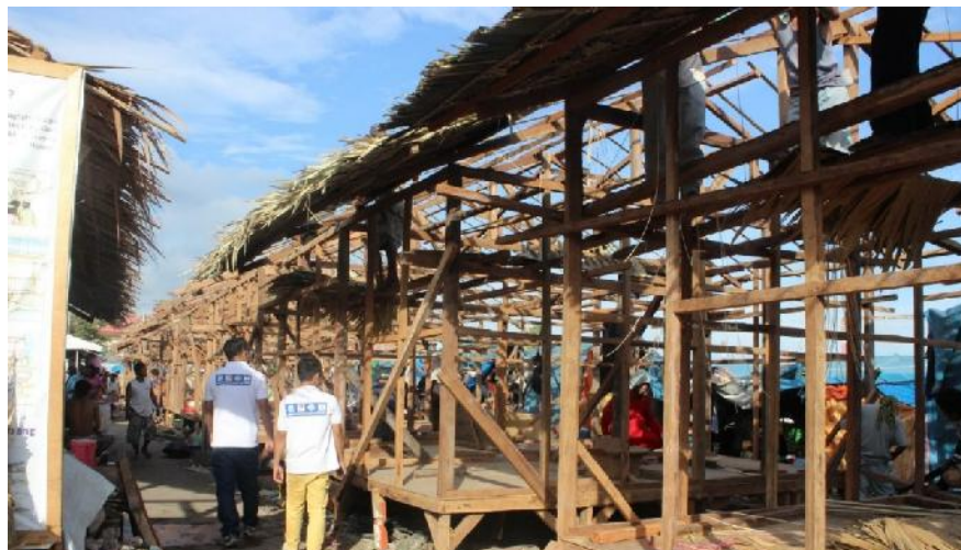
Construction of elevated quadruplex rooms with nipa roofing is ongoing in Zone C.
