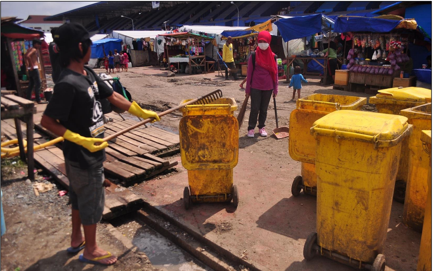
IDPs in Grandstand do regular cleaning of the drainage system as part of the Cash for Work Livelihood program.
